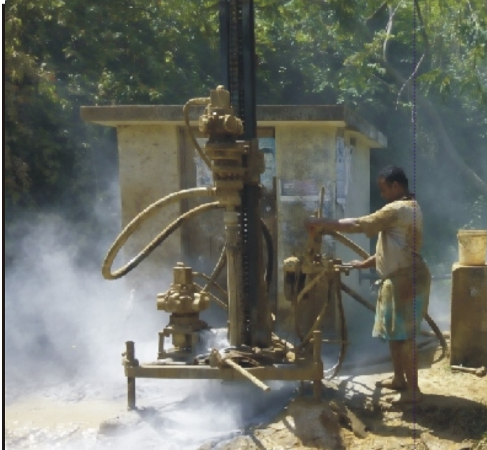
Source Development Bore well @ Peradipallam
